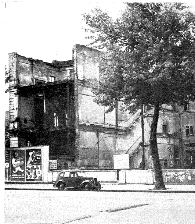
Site of Baden-Powell House prior to the demolition of bomb damaged buildings in 1959.
